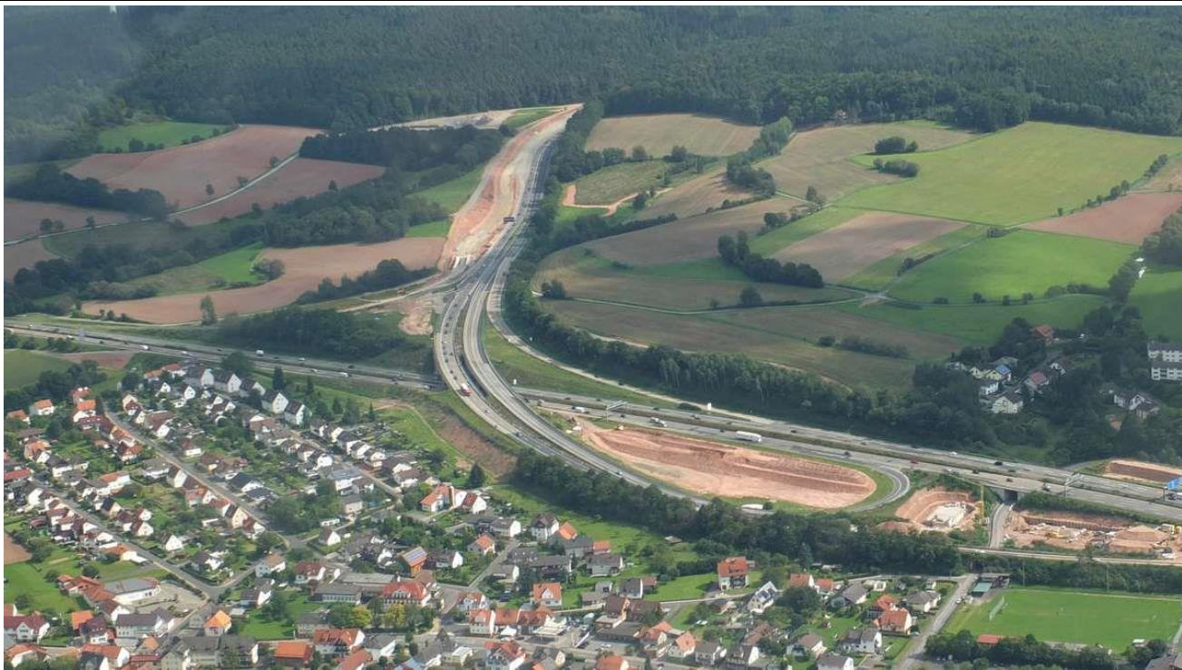
A view of the Kirchheim autobahn intersections under construction in December, 2017. This view is approximately east, towards Bad Hersfeld, along the A-4. The A-7 runs left-to-right in this photo, with north to the left edge. There would have been more vegetation here in the mid-1980's. The autobahn would not have been as wide as is seen here.
